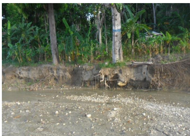
Erosion of the Bainet River bank
