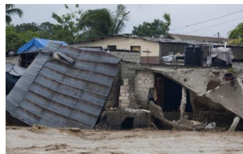
Damage in Haiti caused by Hurricane Sandy
