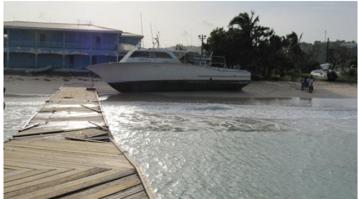
Damage to police jetty in Anguilla as a result of the passage of Hurricane Earl
