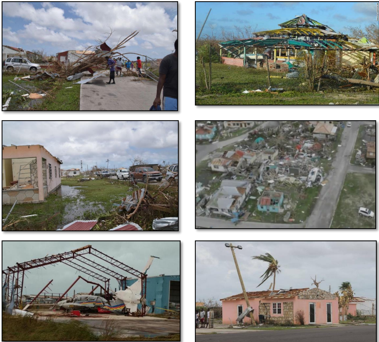
Figure 11 Damage caused by Hurricane Irma in Antigua and Barbuda – September 2017. Sources: Cable News Network, The Telegraph and The Weather Channel
