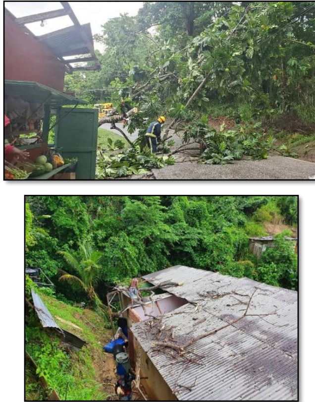
Figure 5 Damage caused by Tropical Storm Gonzalo in Trinidad – July 2020. Source: Ministry of Rural Development and Local Government
