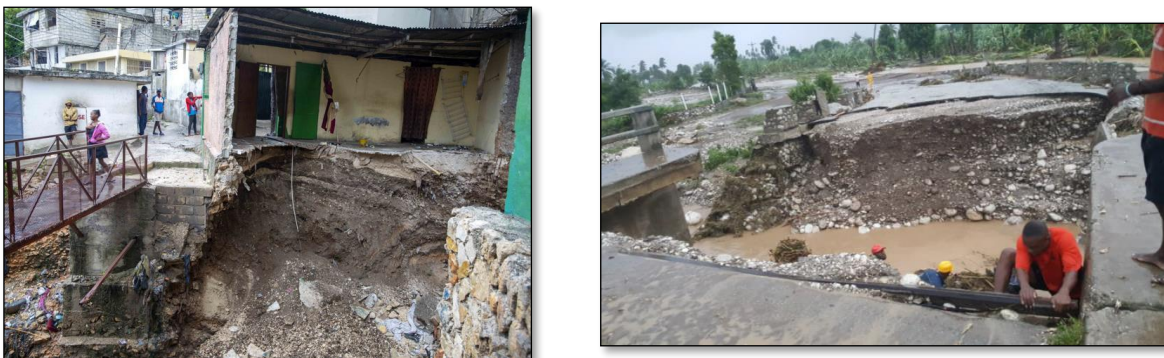
Figure 3 Flood damage caused by Tropical Storm Laura in Haiti – August 23-25, 2020 Source: New Orleans, LA Local news, Voice of America and CBC/Radio-Canada
