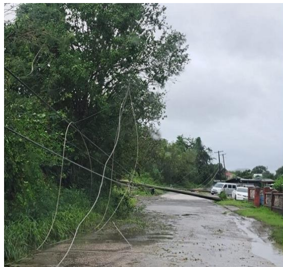
Downed power lines
