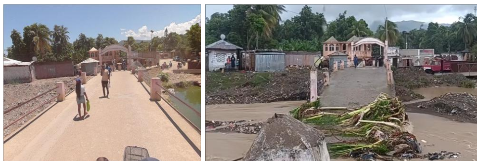
Figure 4 Before and after the destruction of Ti-Rivière bridge 6
