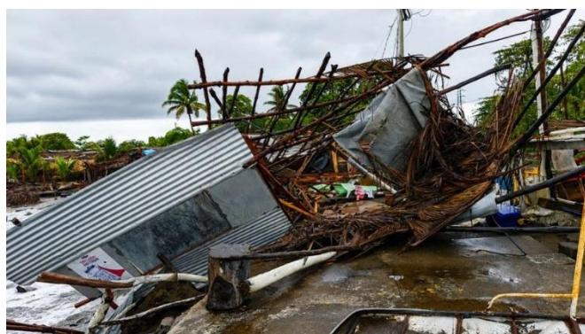
Figure 5 Coastline damages in Paso Caballos, Corinto, Nicaragua. Source: Corinto Mayor's Office FB
