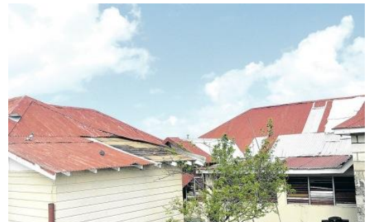
Damage to the Muirton Childcare Facility following the passage of Hurricane Sandy in October 2012
