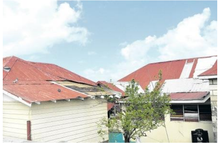
Damage to the roof of the Muirton Childcare Facility following the passage of Hurricane Sandy in October 2012
