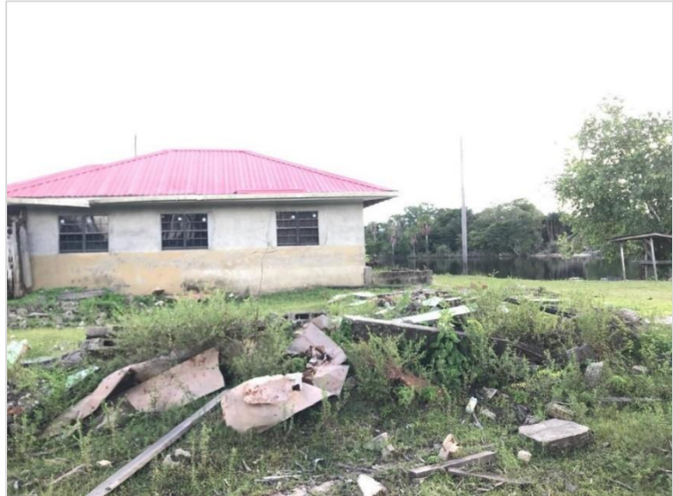
Figure 5.8 Indicating the height of flood water reached during the 2021 flooding event (main river in the background).
