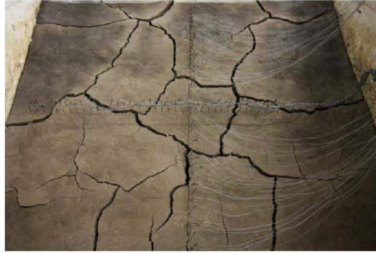
Figure 2-12: Desiccation cracks on a scaled clay embankment after a drying cycle (Khandelwal, 2011)
