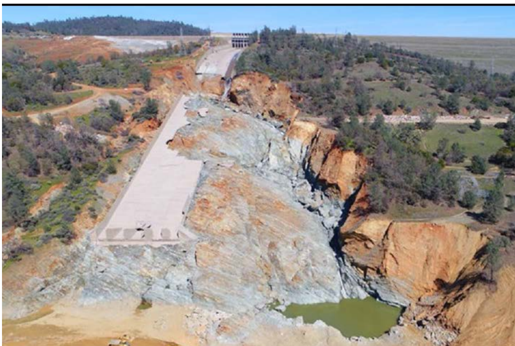
Figure 2-22: Oroville dam spillway damage (Oroville Dam Spillway Incident Independent Forensic Team (IFT), 2018)
