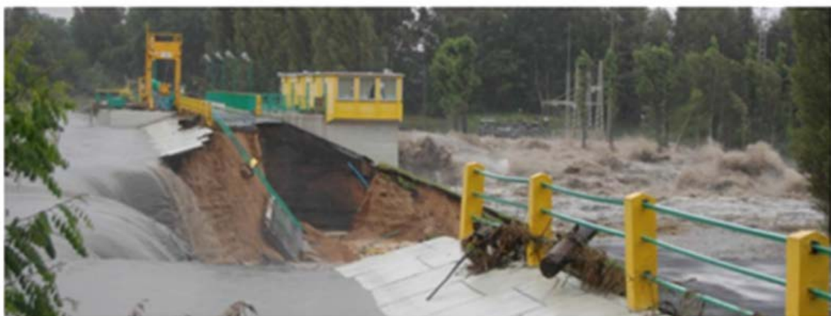
Figure 2-21: Niedow Dam Breach Failure (Kostecki & Banasiak, 2021)
